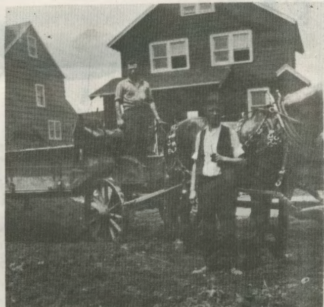
ROAD CONSTRUCTION - in Teaneck in 1925. The worker standing by the horse is the late George Fuchs. Photo courtesy of Mrs. M. Reilly (Fuchs) of Teaneck.
